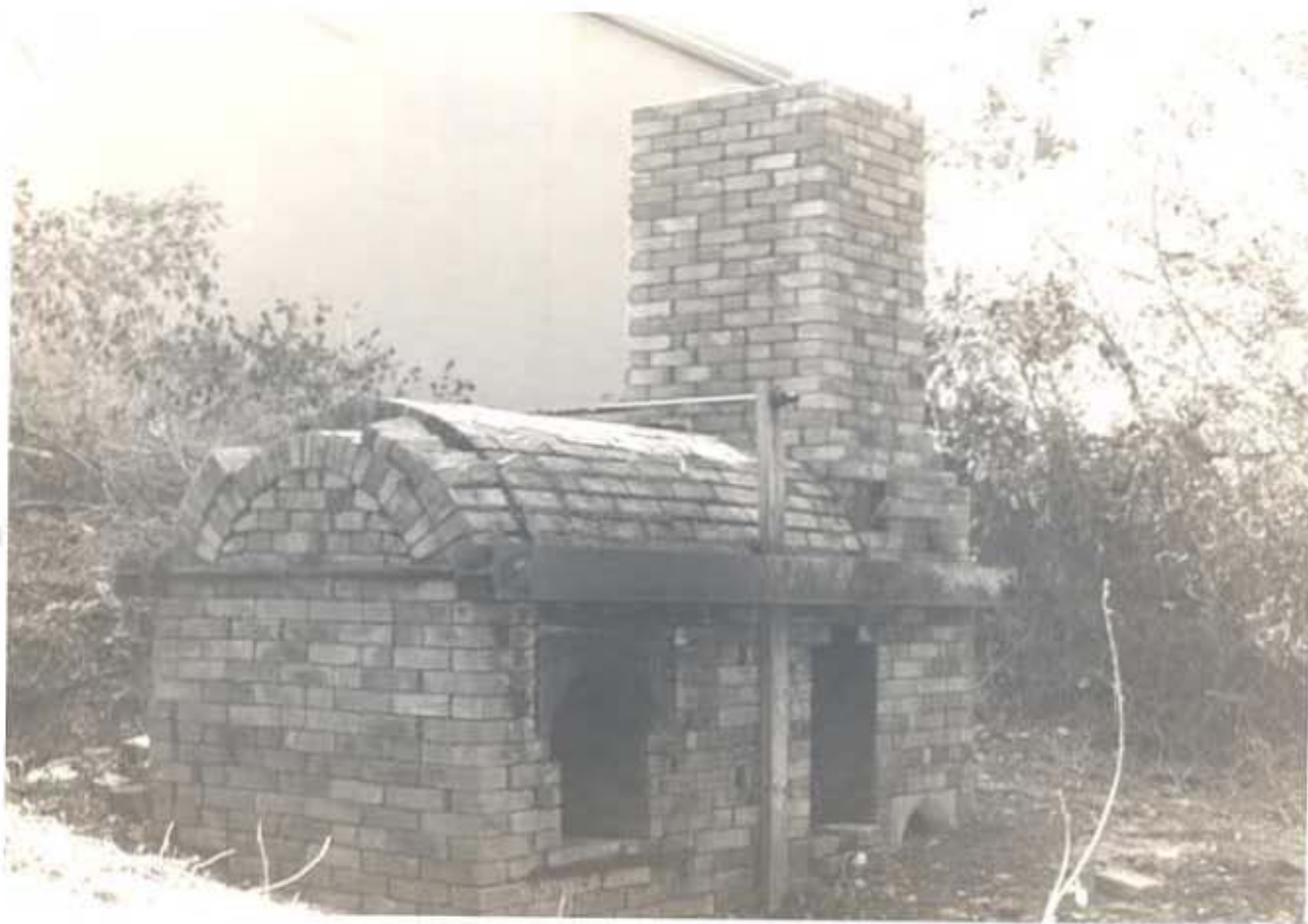
PINEWOOD POTTERY BEFORE RESTORATION Constructed and operated by Converse and Edith Harwell 1939 - 1964 Present owner Eastern Shore Art Association Fairhope, Alabama
