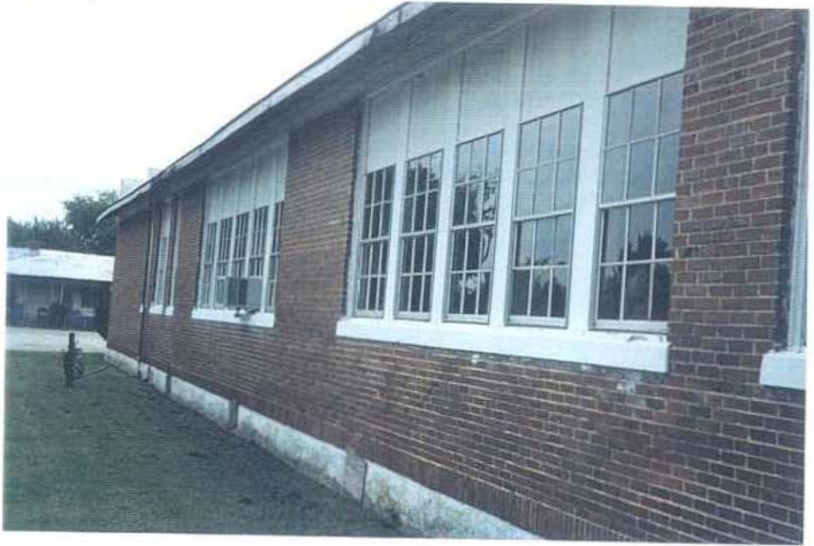
Outside view of 8, 9, 10 & 11 th grade room win- dows and kitchen North sides of LTS
