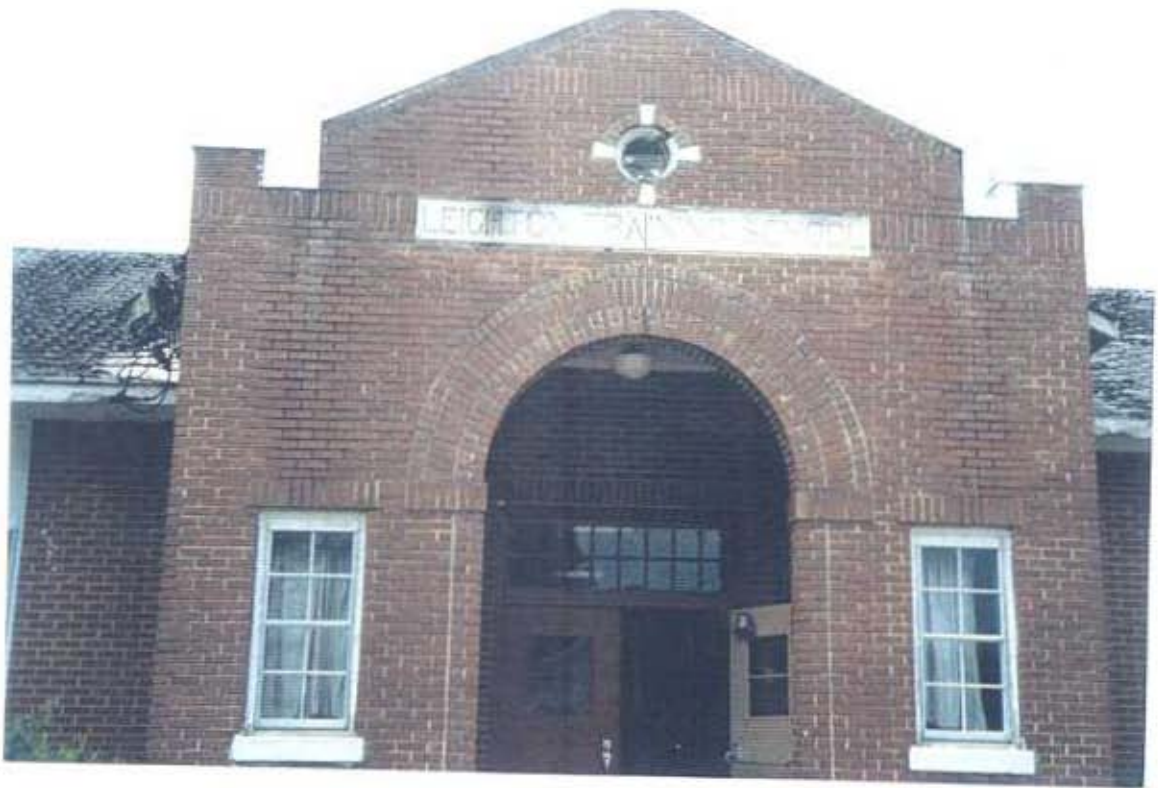
Front entrance of LTS showing roof in state of disrepair 8-12-93
